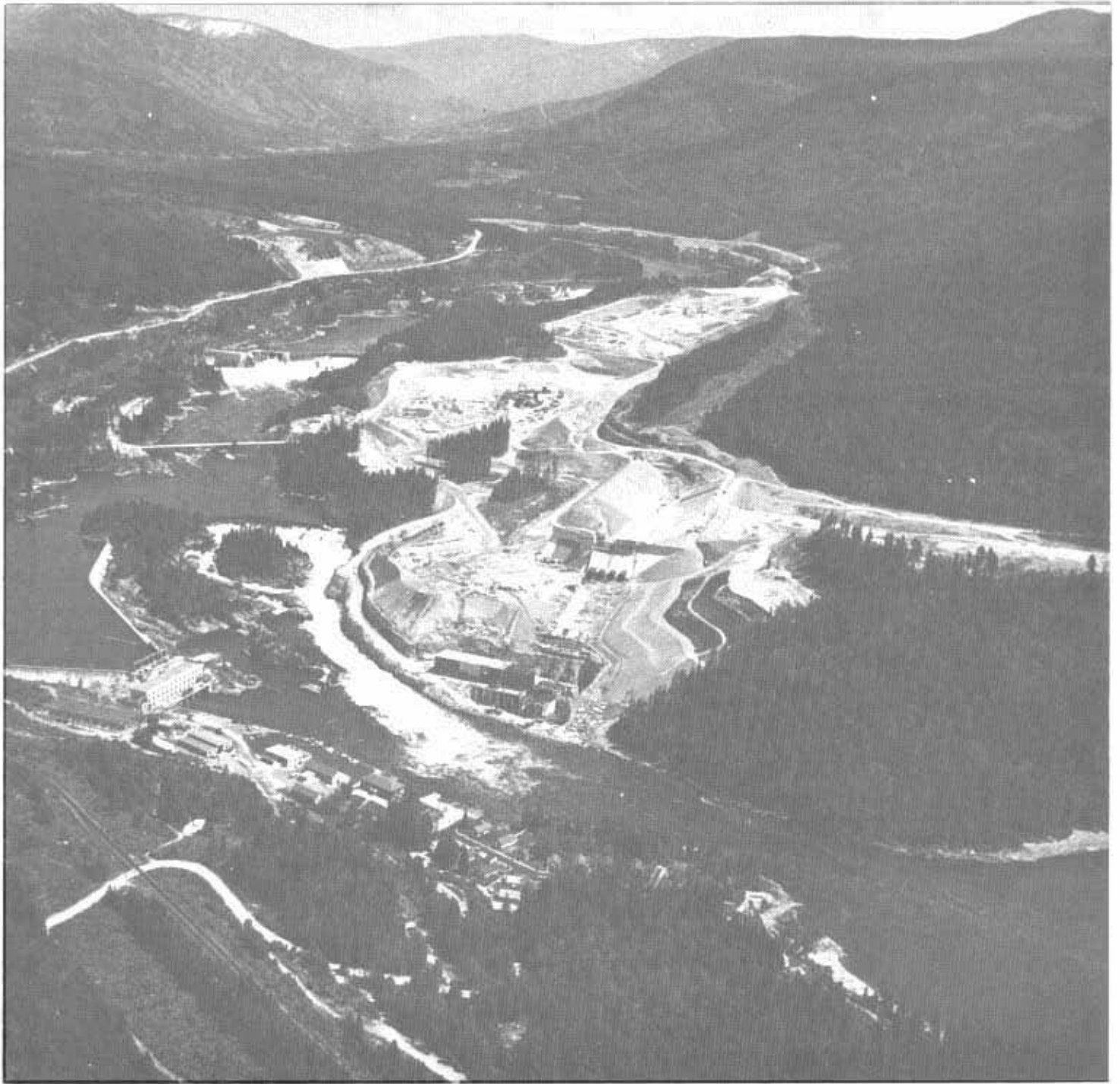
View of Kootenay Canal project construction as of May 1974. The upstream end of the canal can be seen along the south bank of the Kootenay River in the background. Near the upper center of the picture is the central pool, and below that is the concrete-lined forebay and powerhouse intake structure. The powerhouse is adjacent to the upper end of the Brilliant pool, in the foreground.
