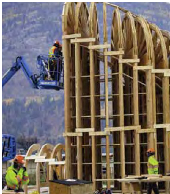
The Waneta Expansion Project is one of four hydroelectric projects intended to help CBT generate a predictable, sustainable and appreciating income stream.
